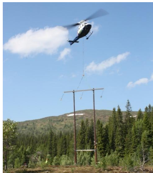
Figure 4 Using helicopter for transport and placing of preassembled poles (Photo: NTE Nett)
