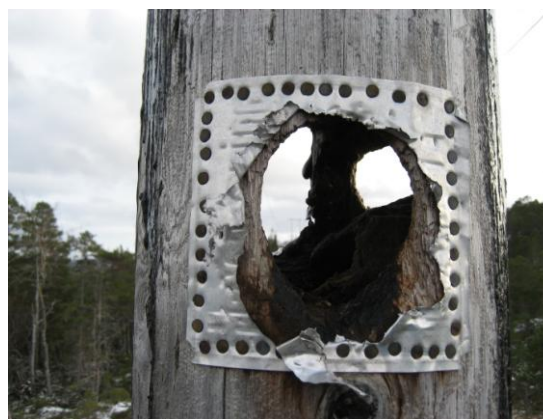
Figure 2 Woodpecker damages on an old pole in the area (Photo: NTE Nett)
