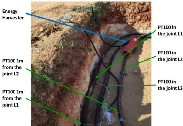
Figure 8: underground installation for monitoring of joints, paper 10797.
