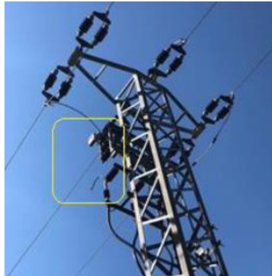
Fig. 6: Phase interruption on the vertical sectionalizer
