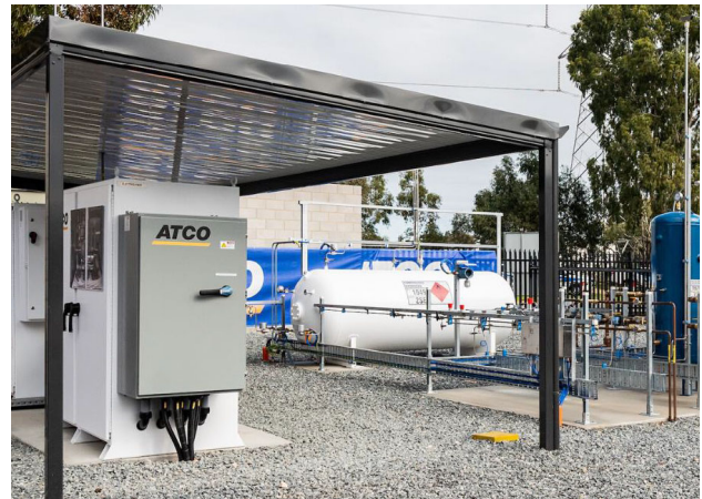
Figure 11. (Paper 0502) 260 kVA controllable hydrogen electrolyser (front left) and 30-bar high-pressure hydrogen storage vessel (centre)
