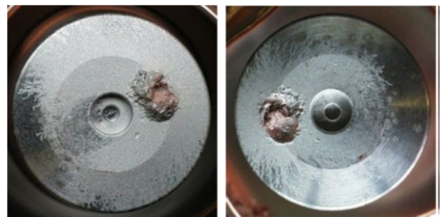
Fig. 2 from paper 1312: Modification of the surface of vacuum interrupter contacts due to making operations.
