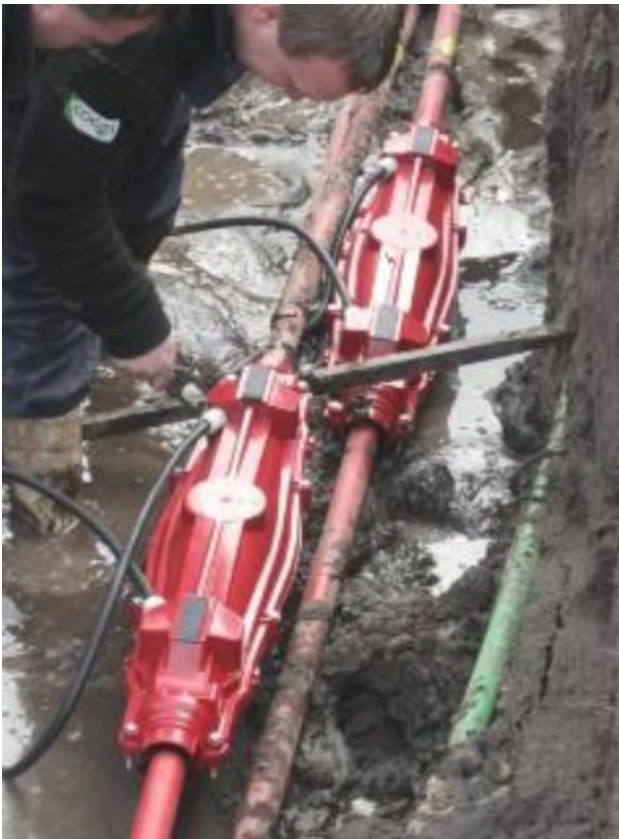
Fig. 6 of paper 0037: Example of cross-bonding retrofitting on MV joints already in service, black bonding wires are visible.
