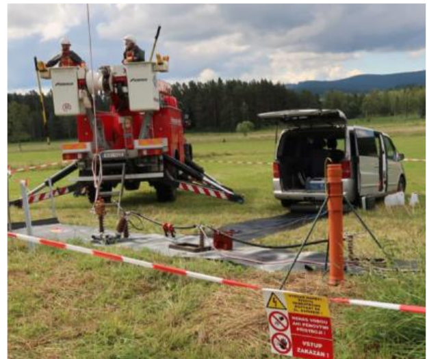
Fig. 28: Preparation of an earth fault ignition (paper 94)
